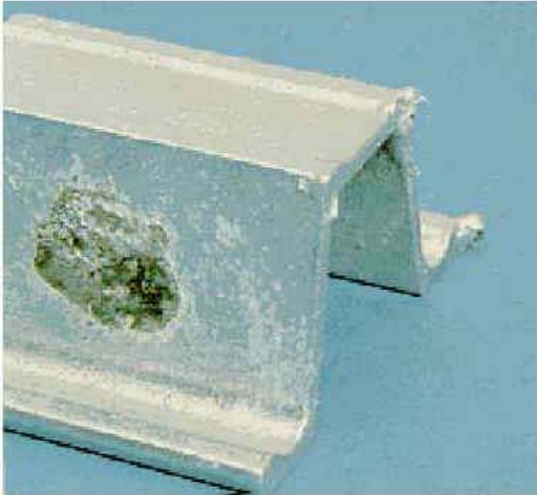
Figure 34-2—Bare (Ungalvanized) Area.
