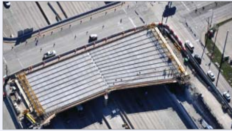
March 2012: Construction of Montfort Road bridge. The first half of the new bridge opens in spring 2012.
