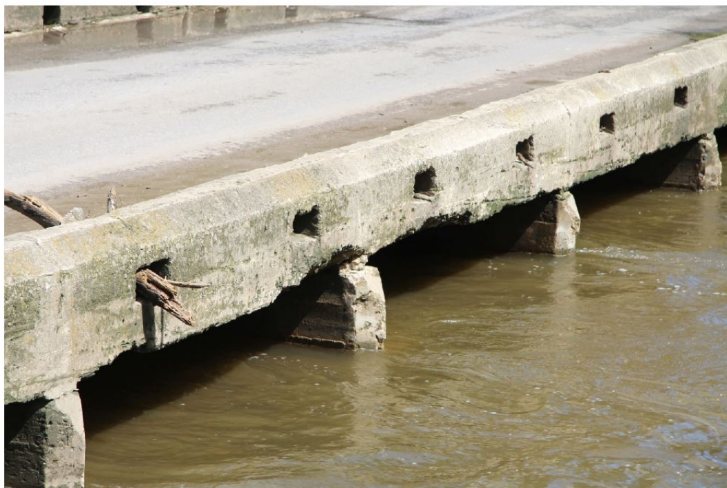
View facing north, showing concrete deterioration on southeast railing, headwall, and culvert barrels.
