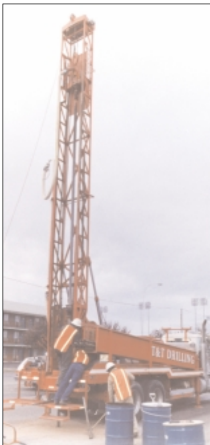
Contractors bore holes to check for levels of gasoline contamination on the Fourth Street storm sewer project.
