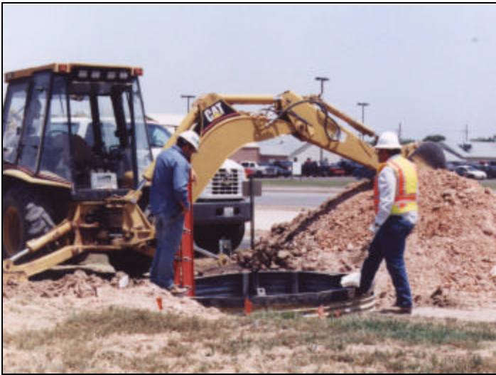
Top and middle photo, Granite Construction Company builds detours in preparation for bridge work at 34th Street and West Loop 289. Bottom photo, city employees take care of utilities off the West Loop access road.
