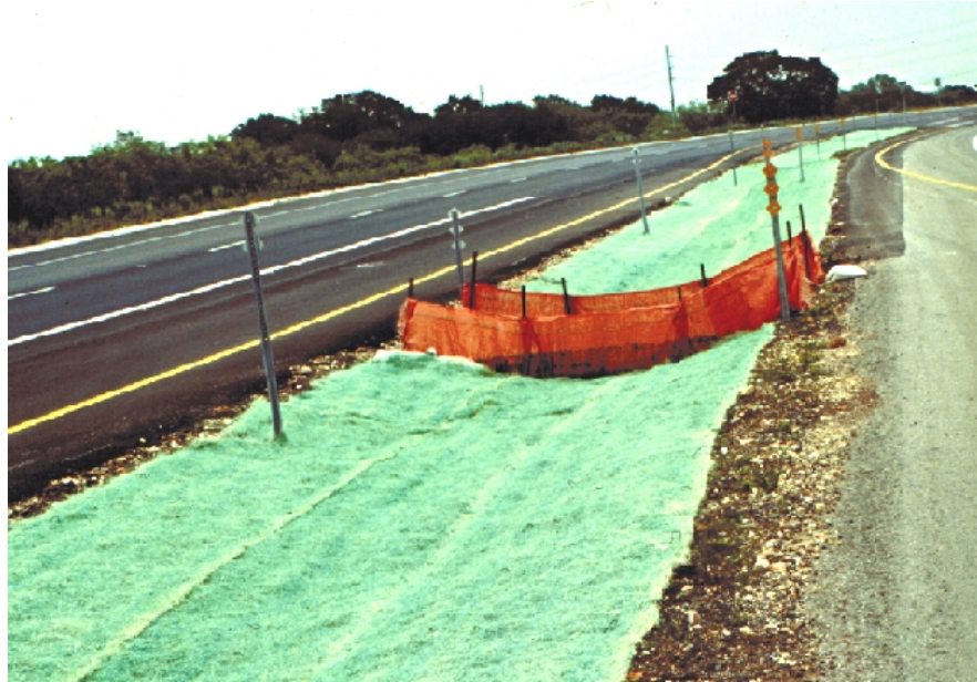
Figure 2.4 - Example of temporary erosion control (matting) and temporary sediment control (silt fence) installed between phases of construction.
