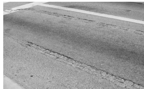
Overlay failure from underlying loop detector sealant problem
